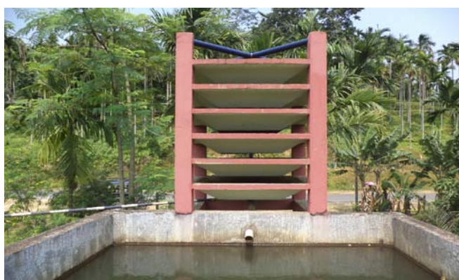
Tray Aerator and Sedimentation Tank of IRP
