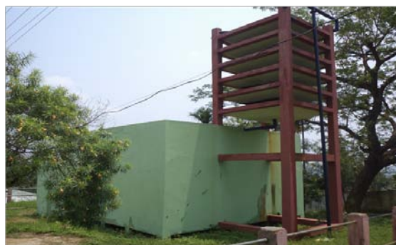
Iron Removal Plant
