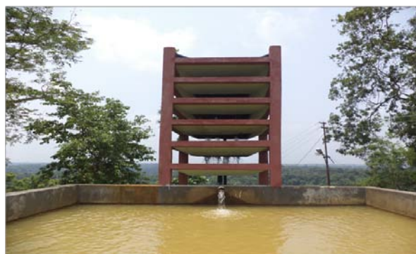
Tray Aerator and Sedimentation Tank of IRP
