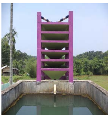
Iron Removal Plant
