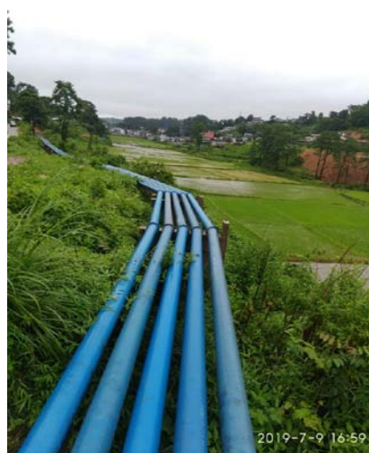
Feeder Main Line
